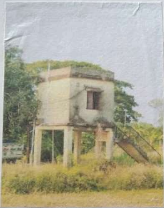
Pic: Water pump house of flooded area
